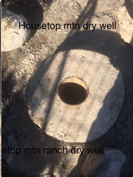
Housetop Mountain Ranch Dry Well
